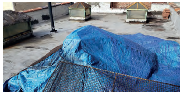
Roof of the sacristy annex at St. Anthony of Padua Church, Bronx NY
